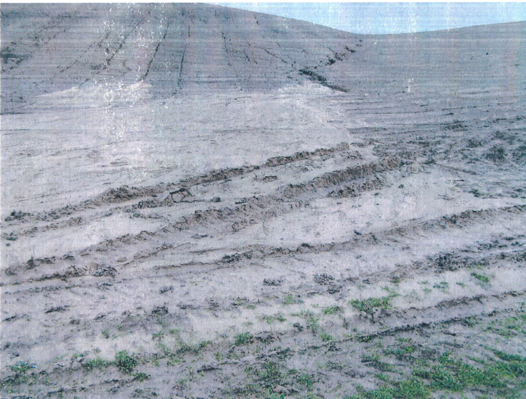
11Jan2008 - Lake Road looking south at eroding graded slope
